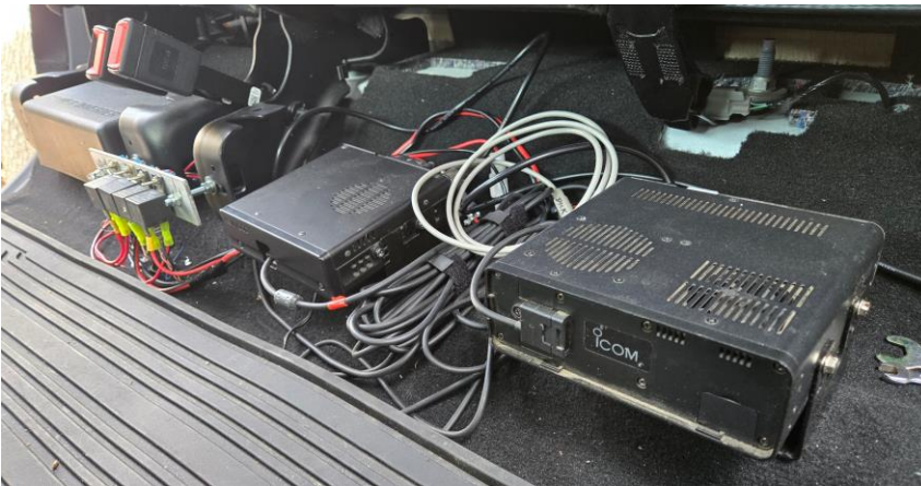
IC-7000 and associated equipment under rear seat
